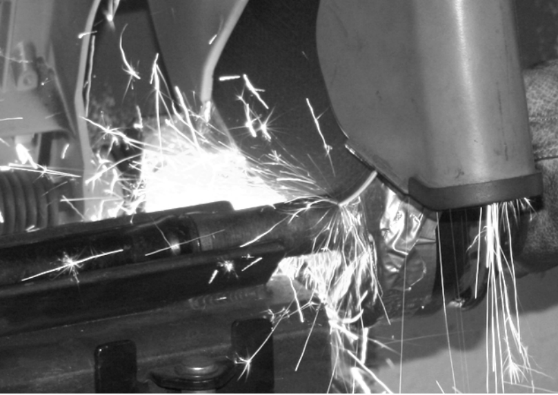
7. Place the axle assembly on the chop saw and cut the axle as close to the joint as possible.
