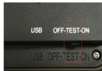
③ Switch to TEST
