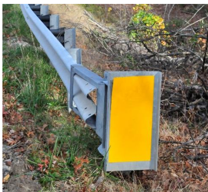
Improper seating of rail into head
