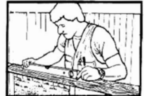
24. Check decks horizontally (trim excavation to suit). Use a level and piece of timber.
