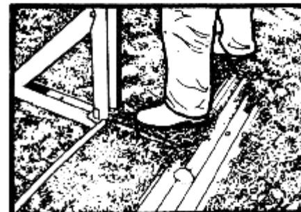
28. Your pool is now ready to concrete. Check vertical levels before concrete hardens and pour concrete into excavated hole to ground level.
