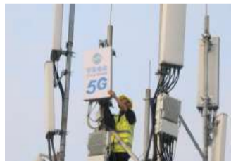
base station back up
