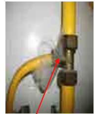
Bubbles indicate gas leak
