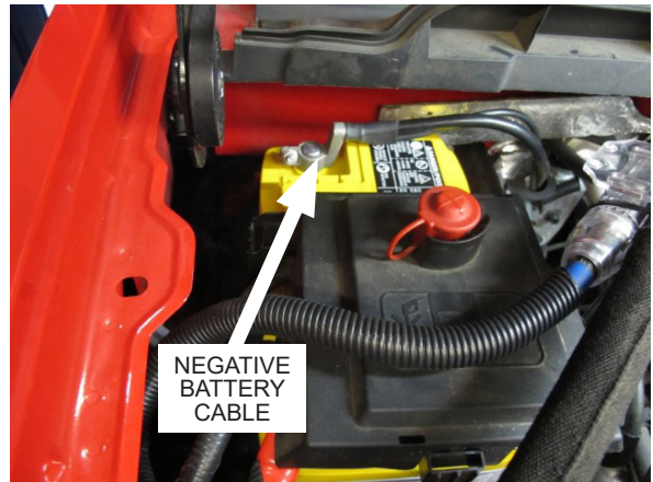
Fig. 13-G: Reconnect negative battery cable
