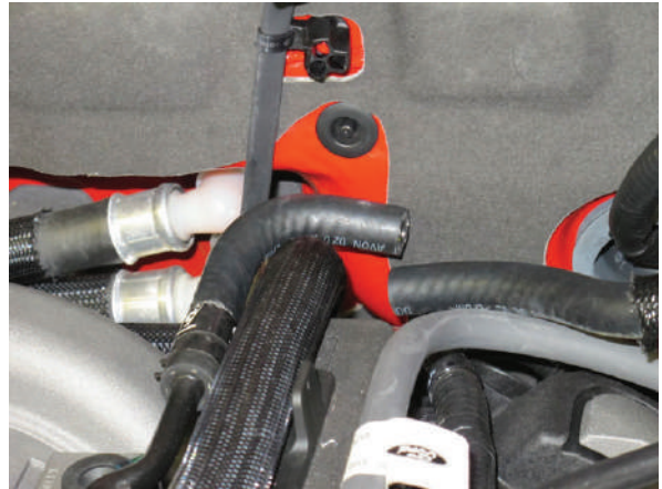
Fig. 8A-1: Vacuum Hose Cut
