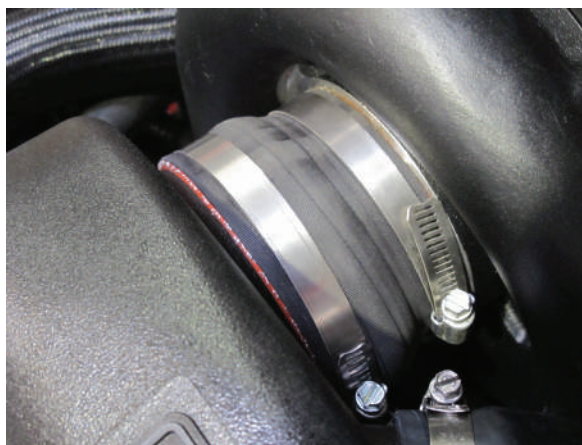
Fig. 11B: Air Inlet to Supercharger Connection
