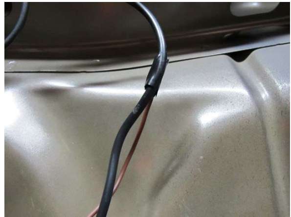
Fig. 6-n: Brown Wire (Unused)
