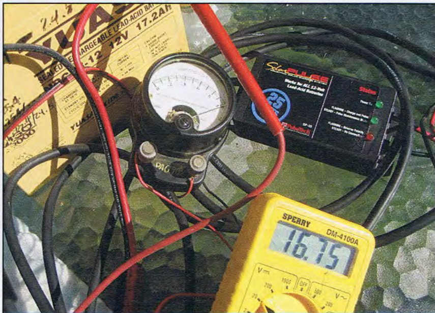
A pulse charger, battery and test gear help tell the story during testing at Quartzfest.
