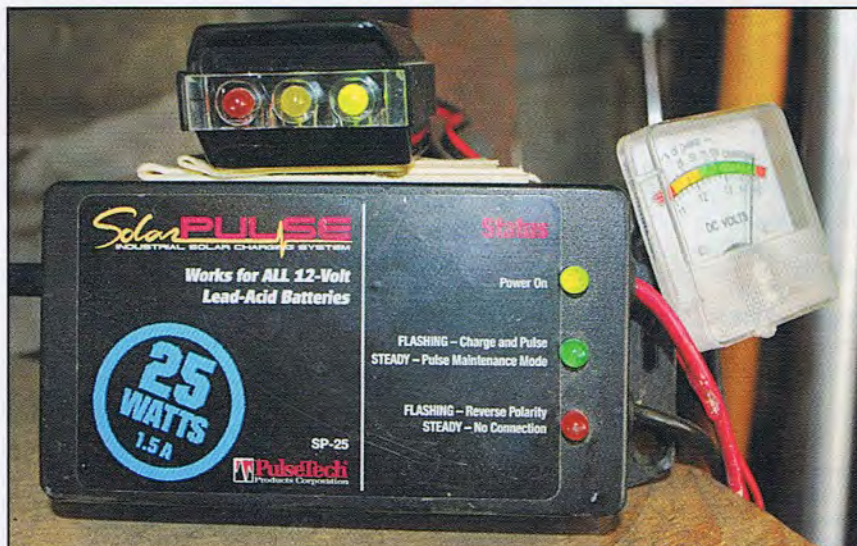
This is a solar panel pulse charger status indicator, with added voltage monitors
