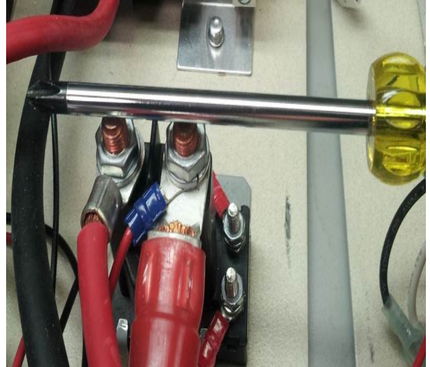
Upright relay failure verification.
