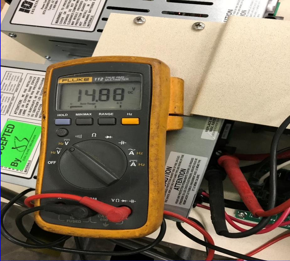
Testing Left side power supply.
