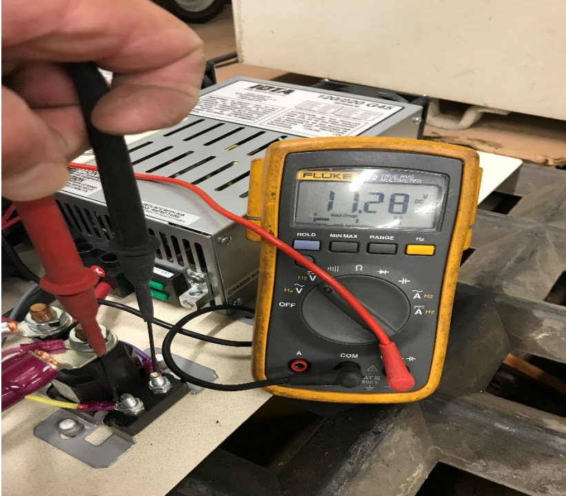
Testing activation VDC on upright solenoid switch.
