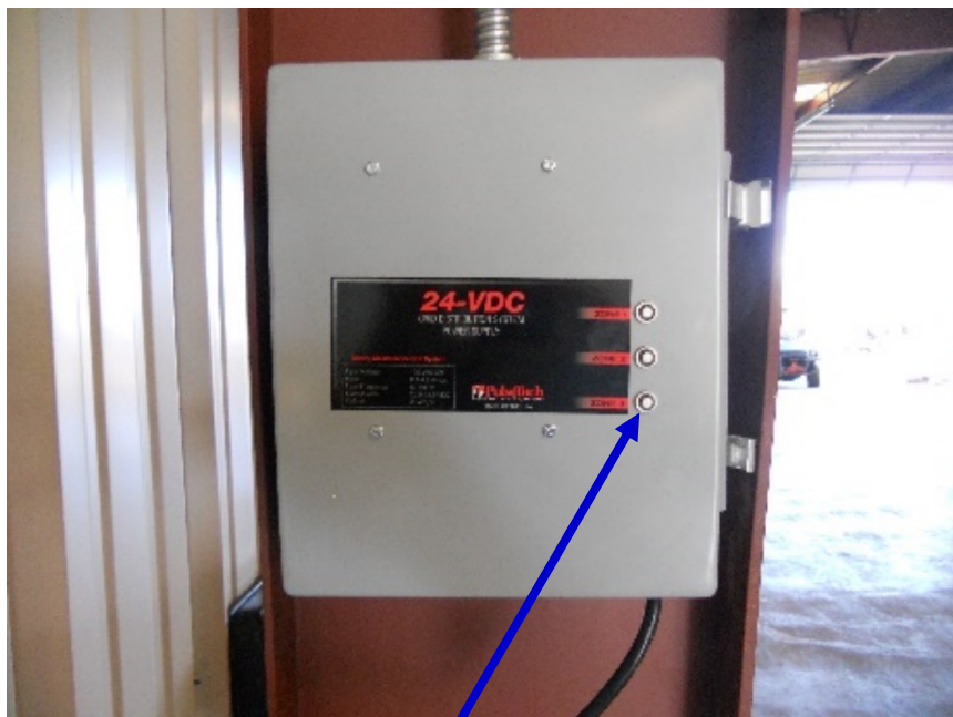
Grid Power Supply – Zone Circuit Breakers
