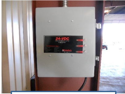
Grid Power Supply
