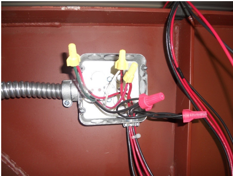
Grid power Junction box.
