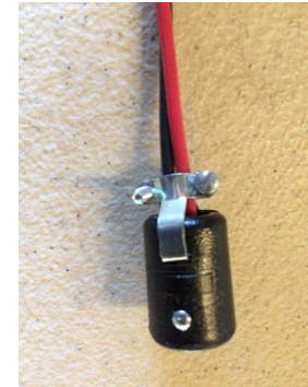
Drop Reel connection harness plug to Drop Reel quick disconnect plug. There should be 30Vdc (+/-) when functioning properly to this point.
