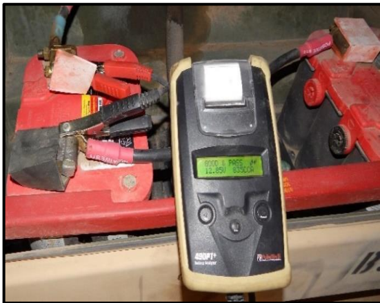
490PT+ being used to test batteries on generator.
