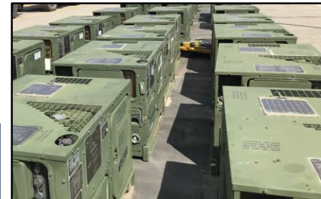
Power generation systems with 7.2 watt panels.
