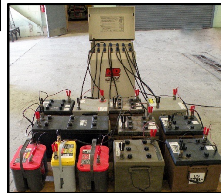
Example: Pallet charger engaging batteries.
