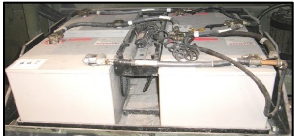
Example: Batteries are series and paralleled with other batteries. There WILL BE CCA and Voltage from paralleled batteries.
