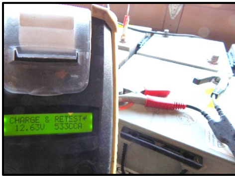
Example: Battery in series / isolated. Tester Results: Charge and retest. 12.6Vdc, 533CCAs
