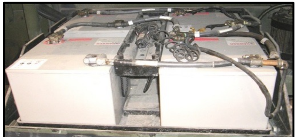
Example: Batteries are series and paralleled with other batteries. There WILL BE CCA and Voltage from paralleled batteries.
