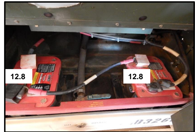
Ready for solar. System is above 24.6 VDC and batteries are balanced.
