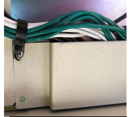
AC wire harness with protective cover.
