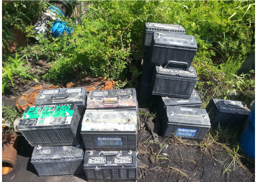
These batteries were thought to be 'dead' and were left outside for over a year.
