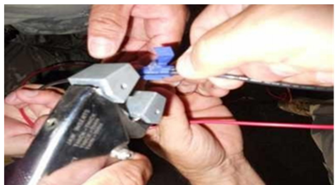
Use the Scotchlok pliers to secure the drop reel harness to the grid with the supplied Scotchloks.
