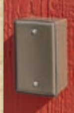
1 Junction Box (mounted on outside of shed)
