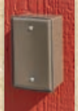
1 Junction Box (mounted on outside of shed)
