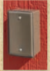
1 Junction Box (mounted on outside of shed)
