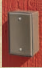
1 Junction Box (mounted on outside of shed)
