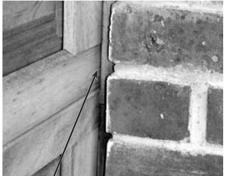
Slight Gap Outside
