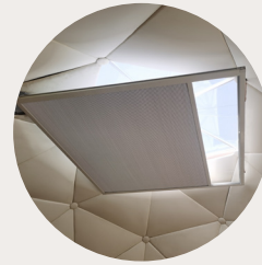
SKYLIGHT MOTORIZED BLIND
