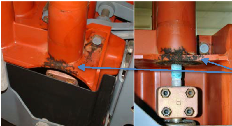
Significant PD Damage
