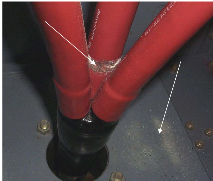
Figure 1 Surface discharge activity between cable phases.
