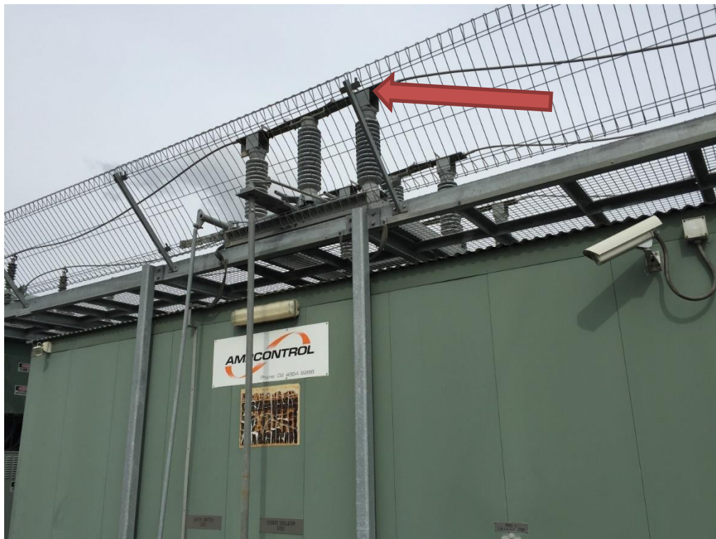
Figure 14 66kV S100 Rotary Isolator
