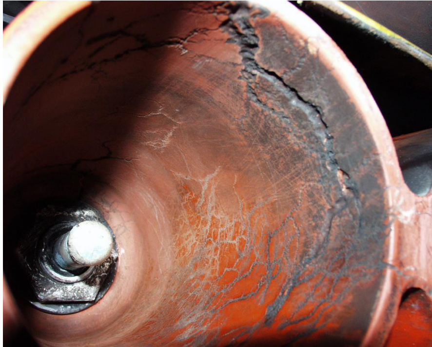
Figure 4 Advanced surface discharge activity within the resin spout of an 11kV circuit breaker.
