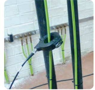
Figure 6: RFCT on earth braid of MV cable - 3 core measurement
