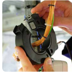
Figure 5: RFCT on earth braid of MV cable
