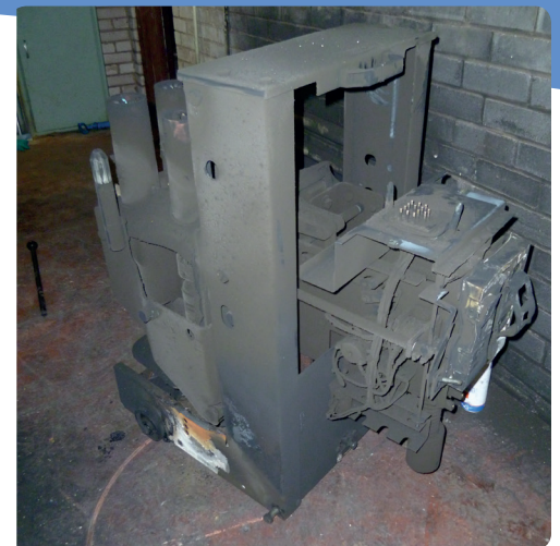
Failed circuit breaker truck
