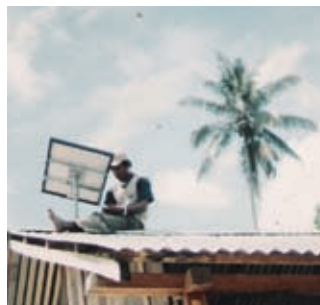
09 Remote solar home systems (50 kWp in Indonesia)
