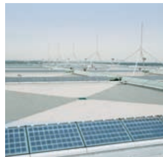
10 Aviation directional lighting
