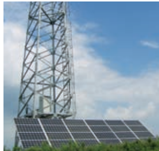
01 Signal transferring station
