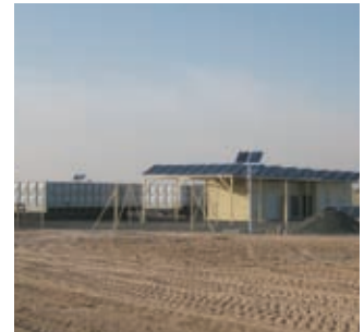
03 43 kWp Solar powered water pumping and desalination system (43kWp in Dubai, UAE)
