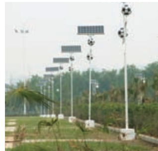
05 Solar powered lights, such as traffic lights, street lamp and etc
