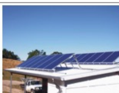
Solar panels in 2 rows
