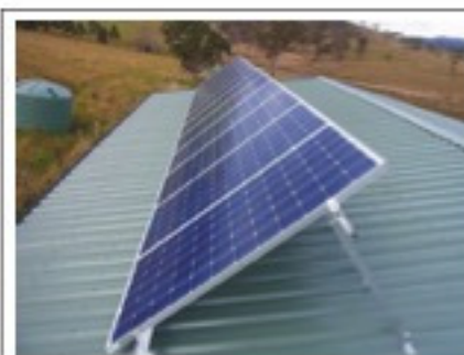
Solar panels in 1 row
