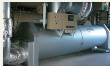
Kagoshima Sendai Plant
