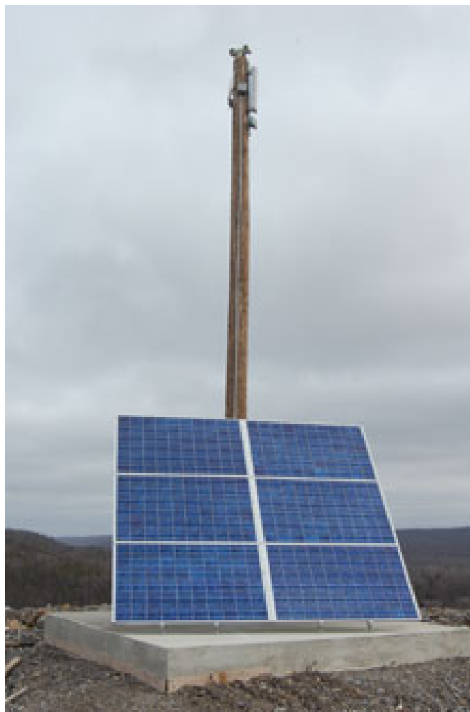
Ground Mount Solar system
