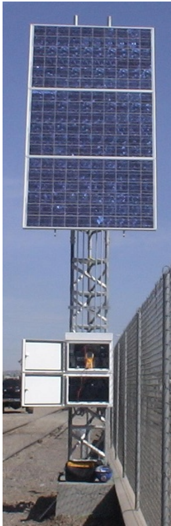
20 Foot tower with Solar
