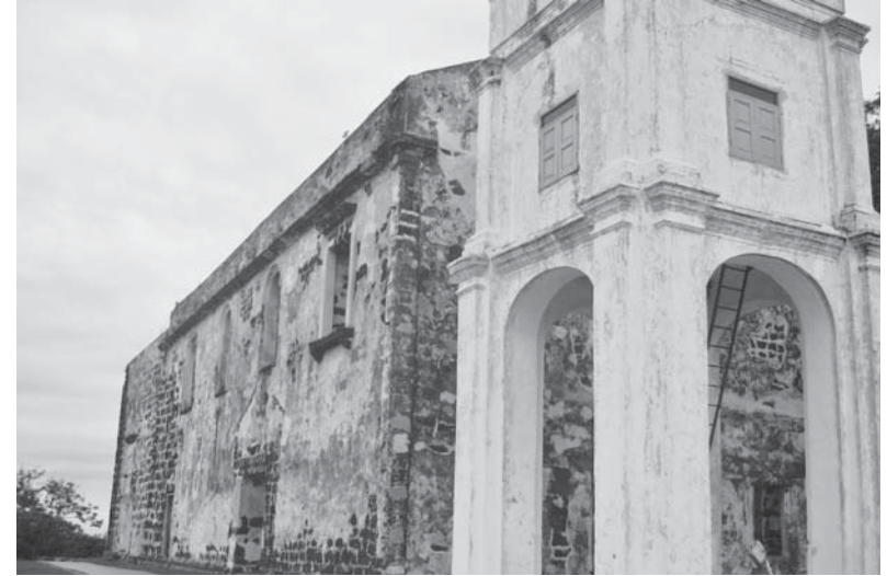
Still standing: the Nosa Senora da Assumpção built, enlarged and consecrated by the Catholic Portuguese between 1521 and 1528. The original building witnessed the bombings and canon-fire in the town below for over 487 years. Note the British lighthouse tower (white). The Malay girl in a tudong entering the old church in the bottom right quadrant gives some perspective of its relative size ©2003 Antonio L. Rappa
