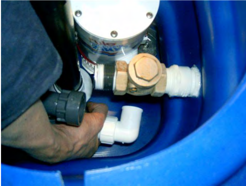
PLUMBING ASSEMBLY REMOVED
