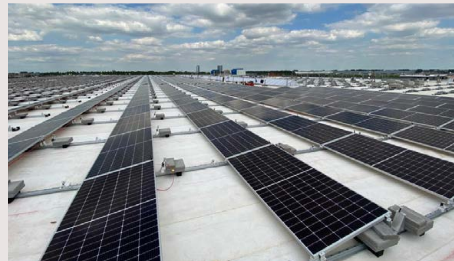
Scotch & Soda warehouse rooftop Hoofddorp, Netherlands - Solar panels
