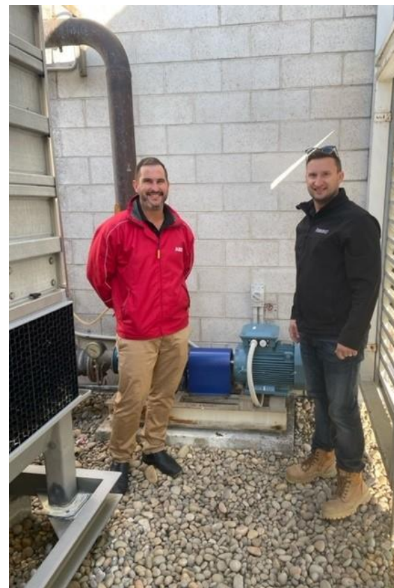
(L-R): Chris Cheong and Tom Green standing beside the chilled water pump and the newly installed ABB synchronous reluctance motor on the plant deck of the building.
