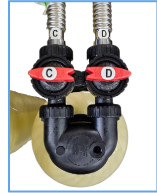
Top view of CT Resin Tank
