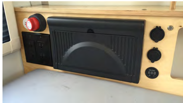
Battery Cut Off Switch / 120V Outlets/ WFCO power center / 12V outlet / USB Outlet / Voltmeter
