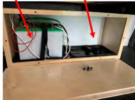
Battery Box – Open Position, (shows one of two battery positions filled)
