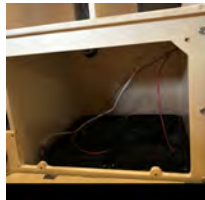
Battery compartment at base of kitchen cabinet – shown no cover, no batteries
