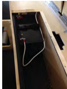
Battery compartment beneath Vberth – shows single battery installed
