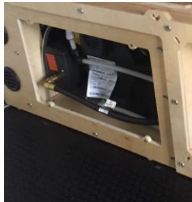
cover plate removed
