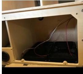
Battery compartment at base of kitchen cabinet – shown no cover, no batteries
