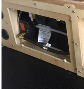
cover plate removed
