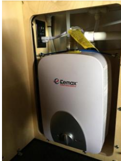
HW heater with storage removed – shows GFCI outlet and connections.
