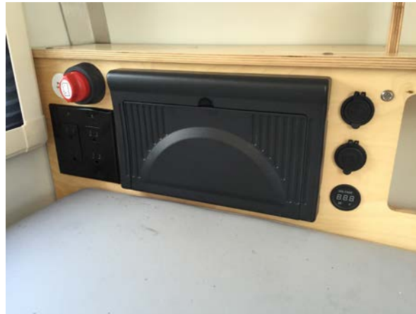
Battery Cut Off Switch / 120V Outlets/ WFCO power center / 12V outlet / USB Outlet / Volt meter
