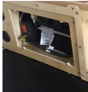
cover plate removed
