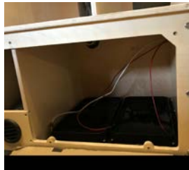
Battery compartment at base of kitchen cabinet – shown no cover, no batteries
