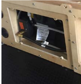
cover plate removed
