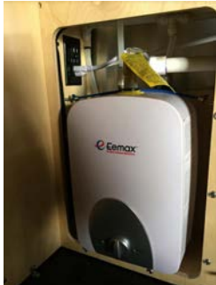
HW heater with storage removed – shows GFCI outlet and connections.
