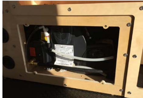
TRUMA location with cover removed.
