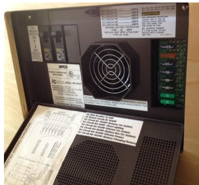
WFCO power center
