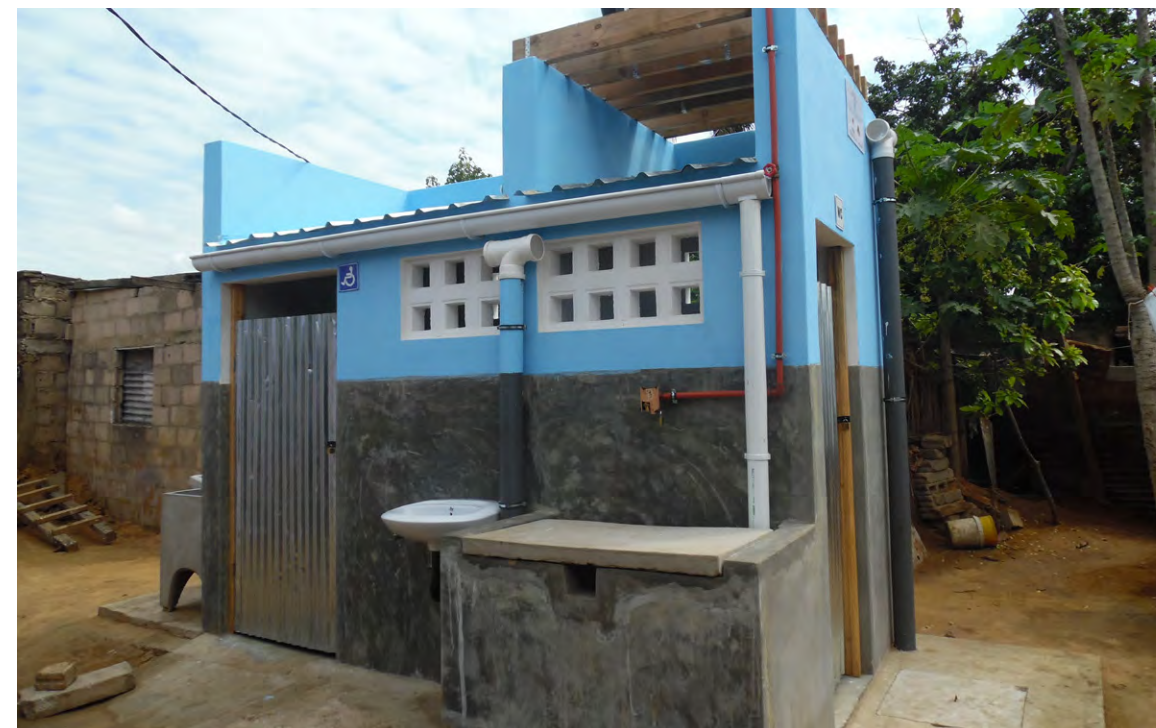
Image: A communal sanitation block in Maputo, Mozambique.
