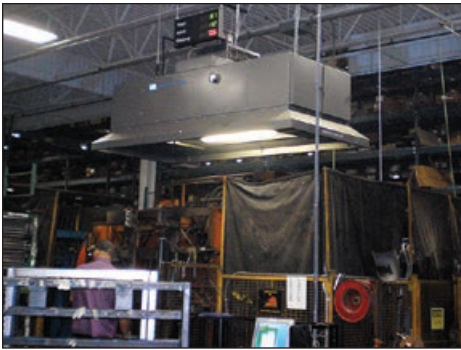
RH35 x 2 - Robotic Weld Cell
