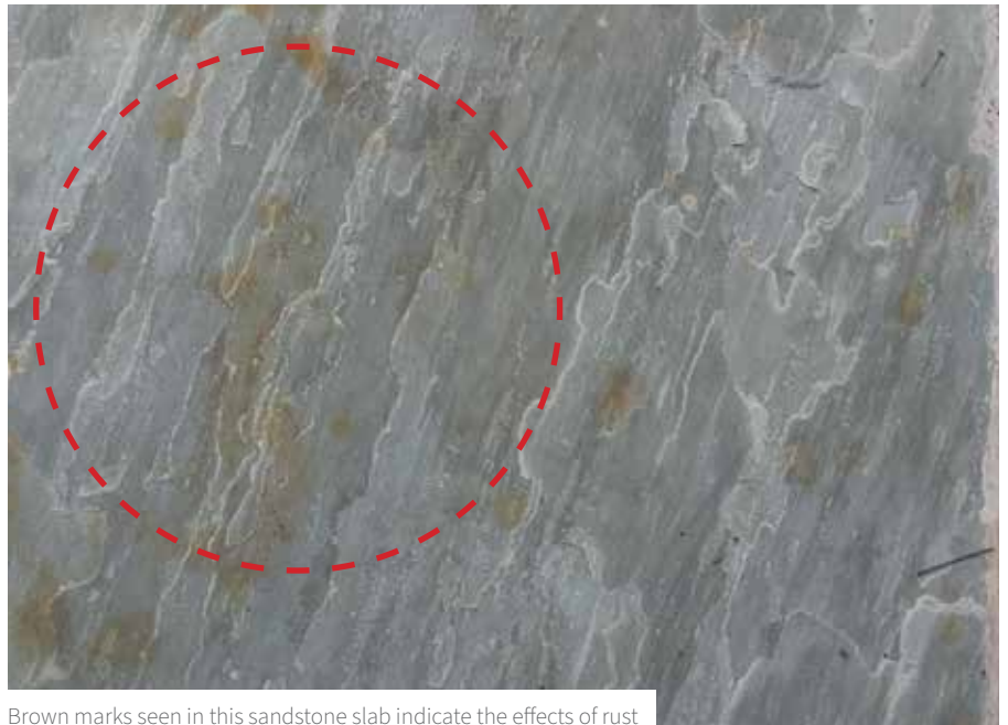
Brown marks seen in this sandstone slab indicate the effects of rust
