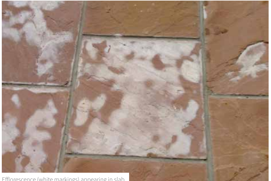
Efflorescence (white markings) appearing in slab
