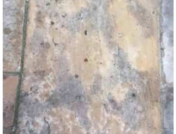
Dark patches showing areas where there are voids underneath
