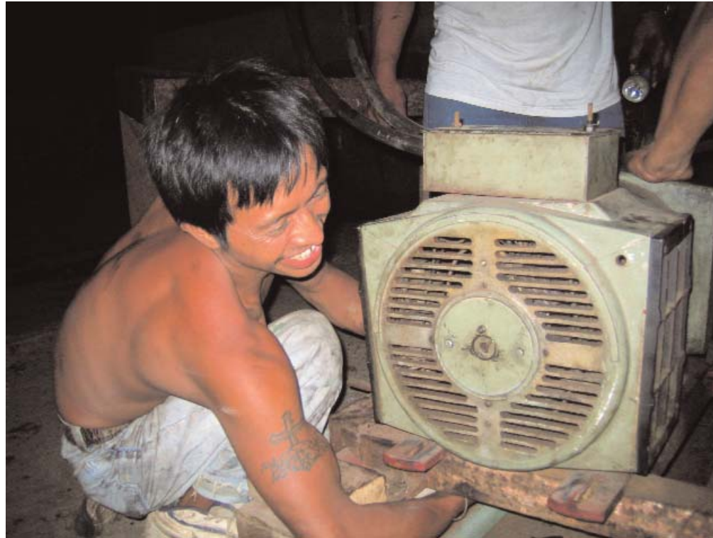
Photographer: Matthew Rudolf Oscar Recinos Chan works in the dark to adjust the position of an electrical generator that has been connected to a biodiesel motor. Work was done by flashlight and with manual tools six days after Hurricane Stan devastated Guatemala.
