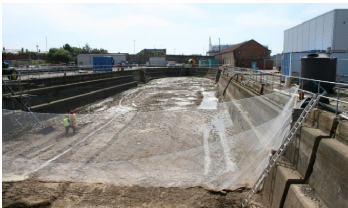
We used a subsea dock including a replica seabed
